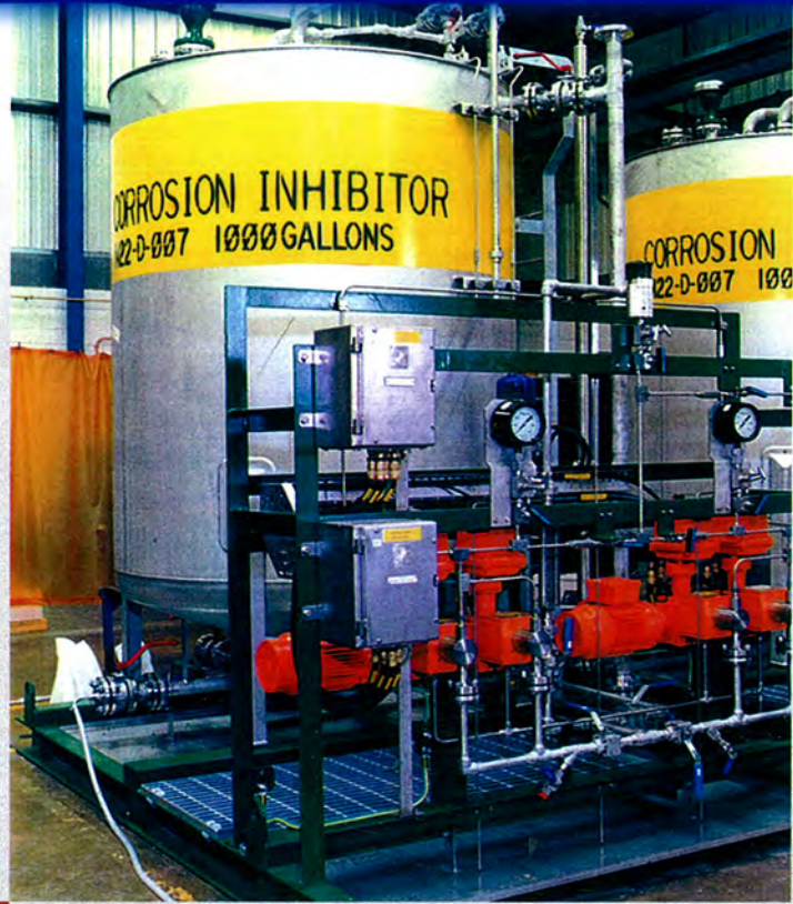
Corrosion Inhibitor Injection Skid
