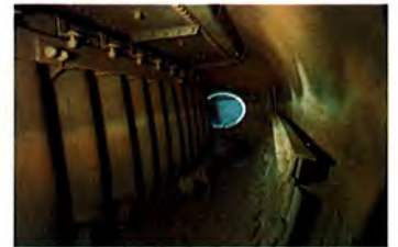
Typical steam drum with generating tube baffle plates, centrifugal separators, and secondary scrubbers
